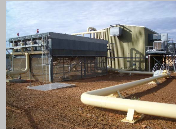
Bulla Park Compressor Coolers
