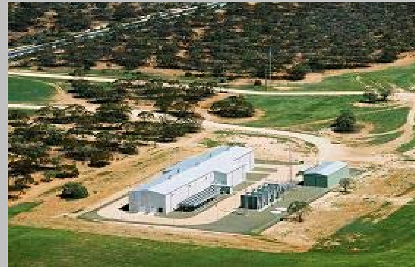
Berri Converter Station
