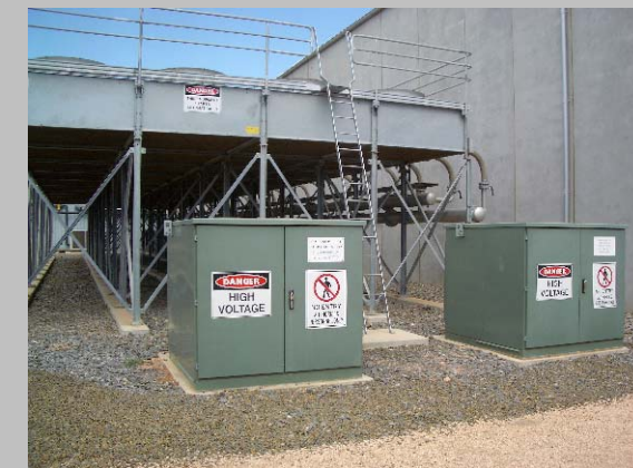
Red Cliffs Station Coolers
