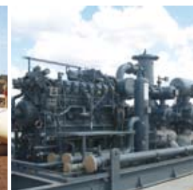
Left: Scraper Station at Bulla Park on the MSP Right: Compressor at Kogan North in Qld
