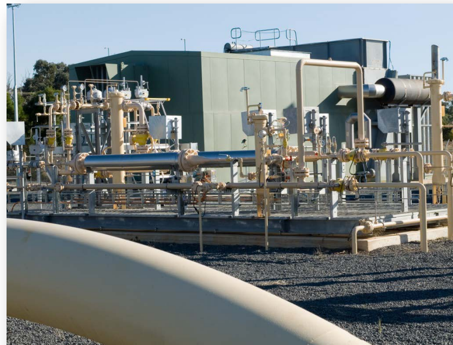
Culcairn compressor station, NSW Enables bi-directional gas flow between NSW and Vic
