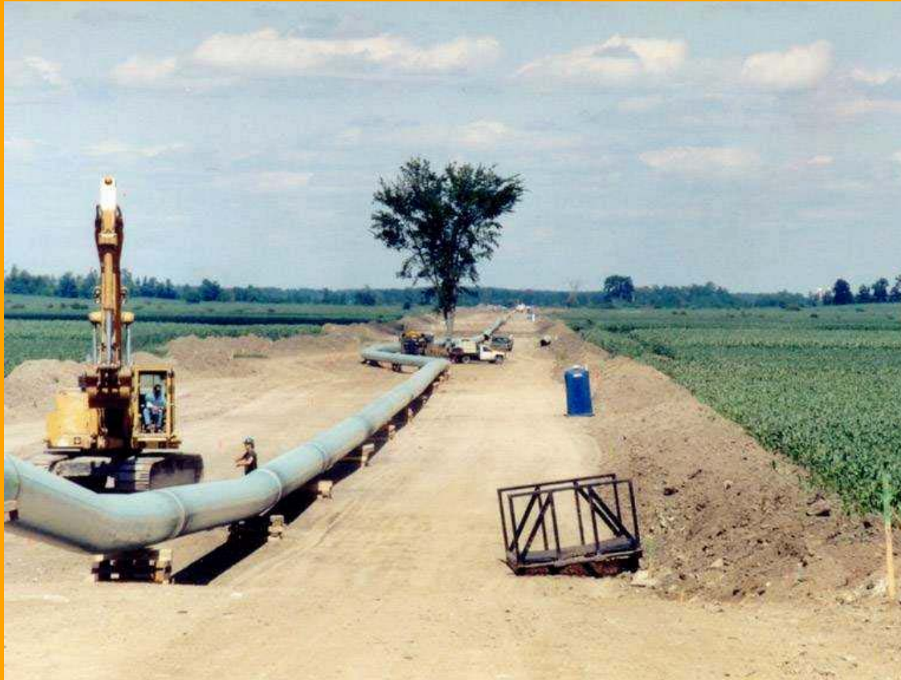
Australian Pipeline Trust – June 2005 APIA Seminar - Meeting New Owners and, Projects and Challenges
