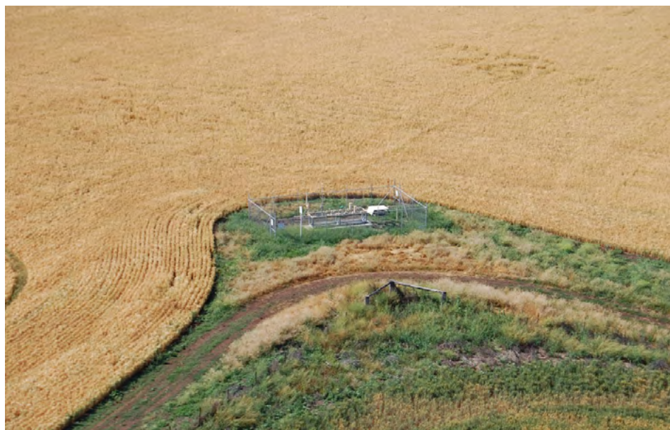
Existing farm tap on the Central Ranges Pipeline
