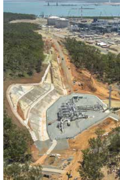
Wallumbilla Gas Pipeline delivery station into QGC's Curtis Island LNG facility
