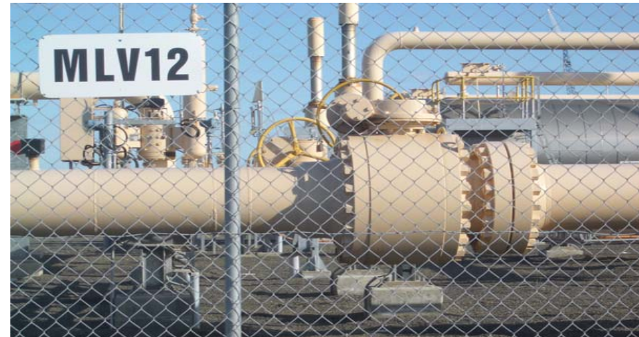
APT AM SEAGas Pipeline
