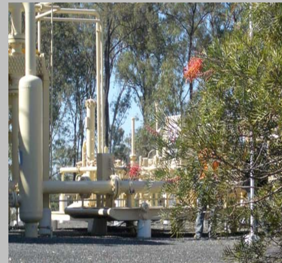
RBP Gatton Compressor Station
