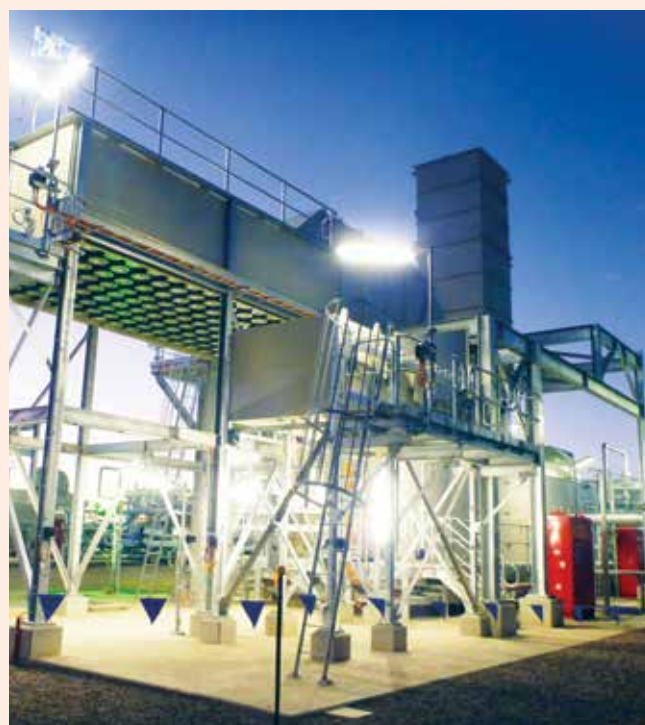
Moomba Compressor Station, South Australia
