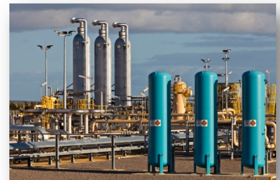
Mondarra Gas Storage Facility
