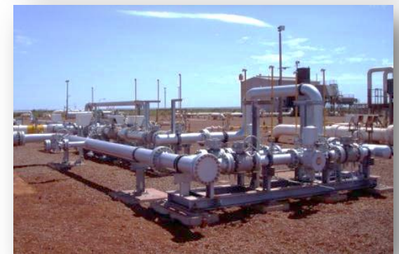
Goldfields Gas Pipeline interconnect with Dampier Bunbury Pipeline - Yarraloola
