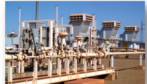
Regulator skid at Newman Power Station
