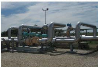
Station reversal skid, Springhurst
